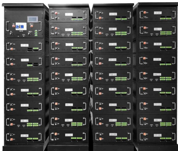
▲ Stack of batteries
